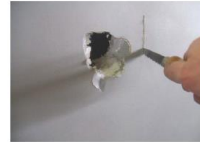
Figure 2: Square Off Damaged Area
