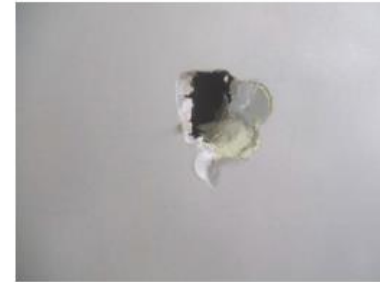
Figure 1: Damaged Gypsum Panel
